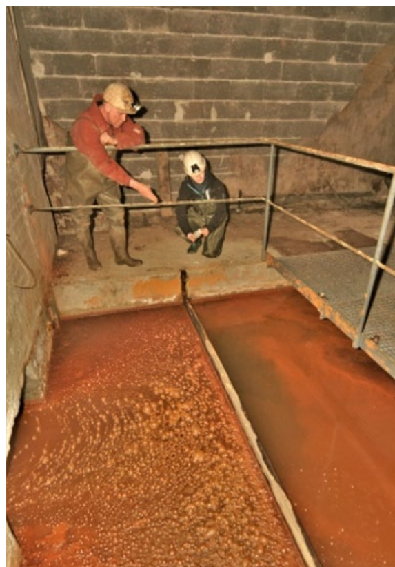
Figure 2: Oil separator at the "Achenbach" shaft in the level of 180 m (m.a.s.l.) "Ernst-August-Stollen".
